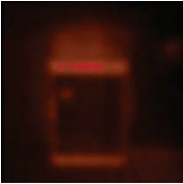
Thermal Image of Cres Cor hot cabinet
